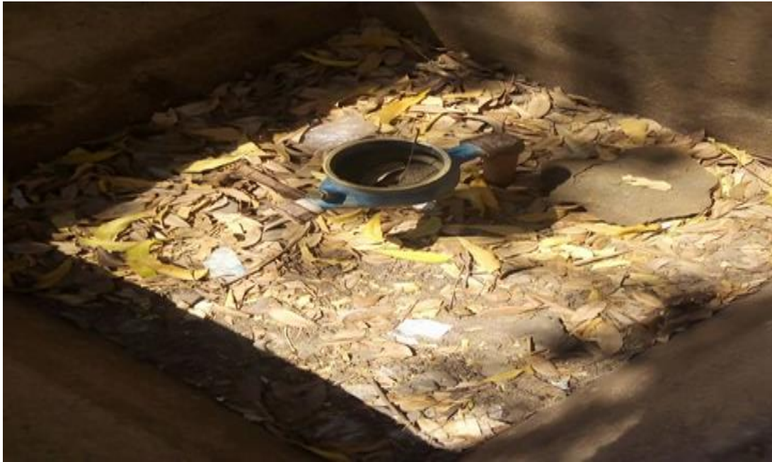
Photograph 1: Non-functional water meter and School D
