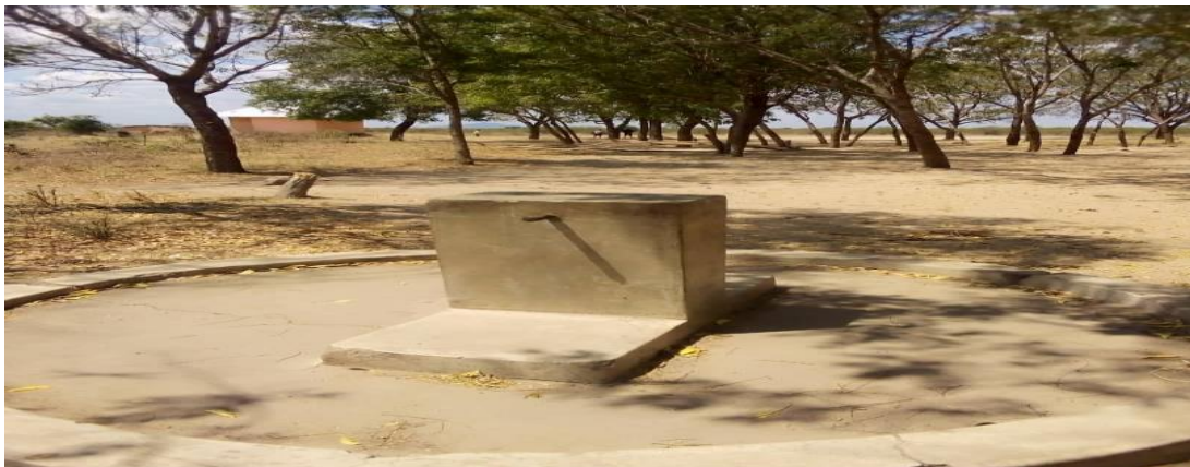
Photograph 2: Damaged hand pump at School D
