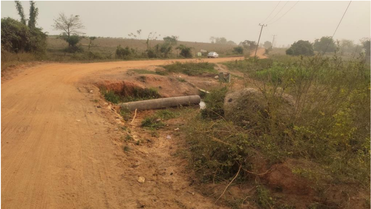
Plate 1: Showing washed off portion on the main road leading to Osogbo farm settlement.
