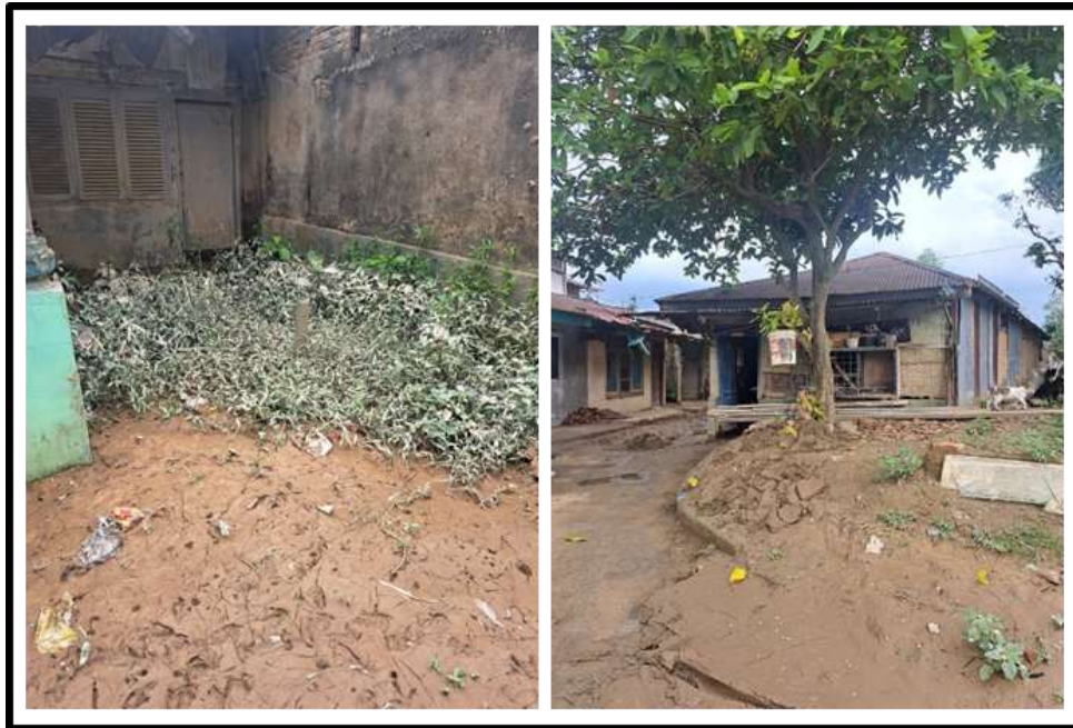
Figure 2: Flood-Affected Wall Condition
