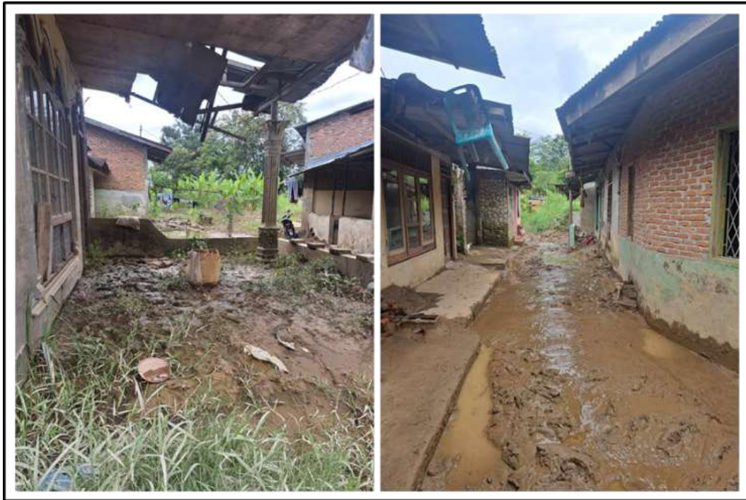
Figure 6: Existing Floor Condition
