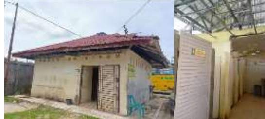
Figure 7: The condition of the toilet
