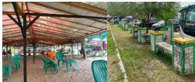
Figure 8: Condition of huts and seating areas
