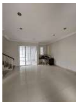
Figure 4.13 ceiling wearing gypsumboard
